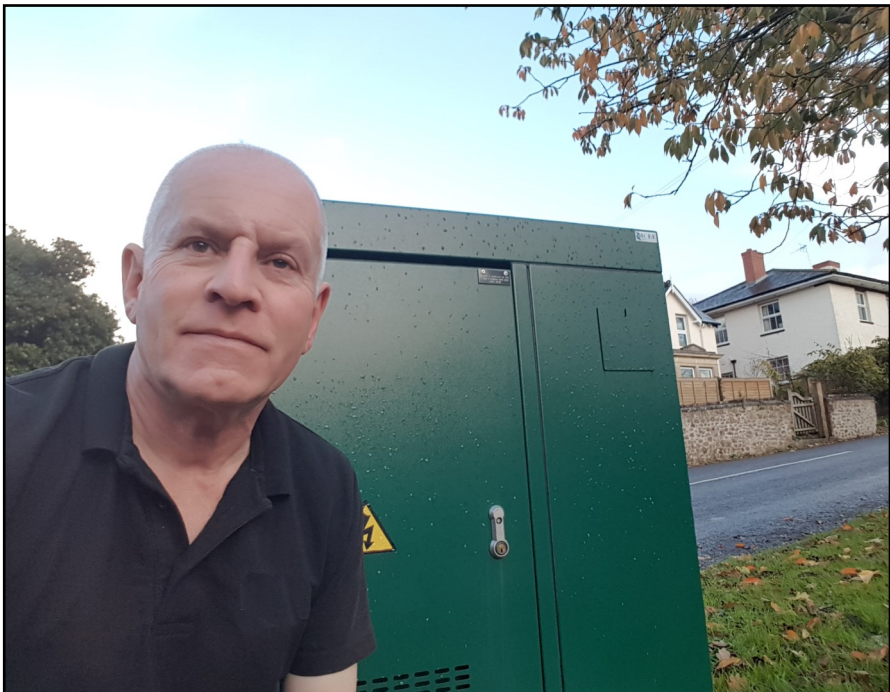
County Cllr John Thorne with a fibre broadband network junction box originally installed by Gigaclear although with the company's branding now removed.
