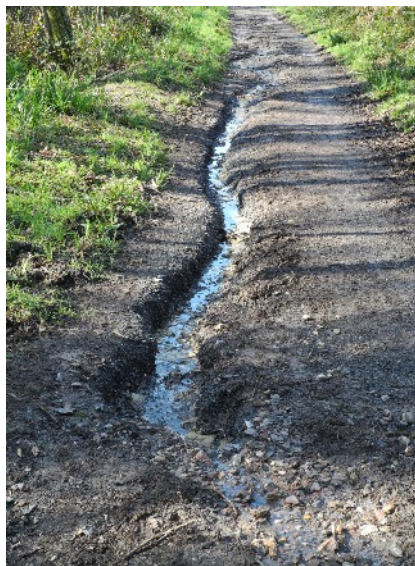
The path before repair
