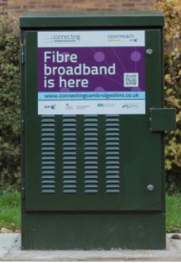
Fibre optic enabled cabinet
